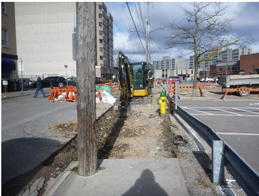
Photo 11: Archaeological Monitoring of the Removal of the Sidewalk Adjacent to Baker Street (Area 2), facing north
