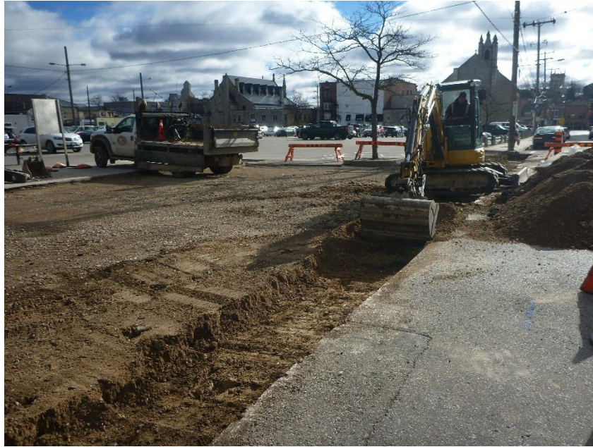
Photo 10: Archaeological Monitoring of the Removal of the Sidewalk Adjacent to Baker Street (Area 2), facing southeast
