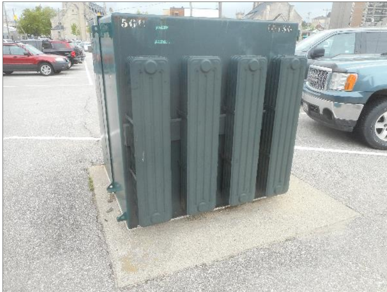
Photo 8 – View of pad-mounted transformer on the east adjacent property to the Site.
