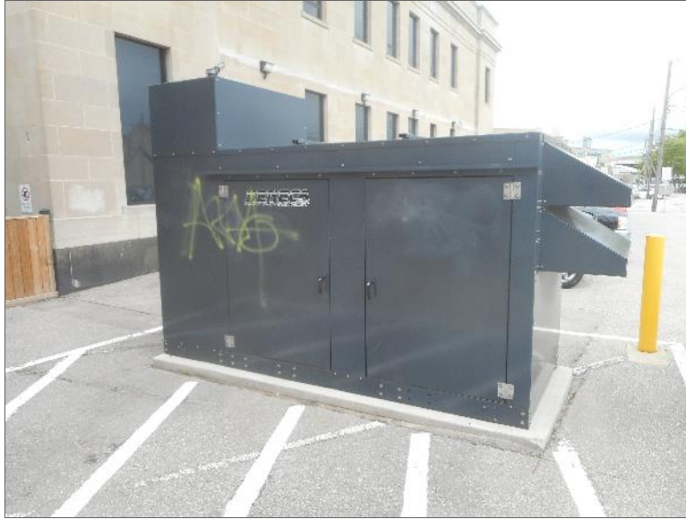
Photo 9 – View of diesel-fired emergency generator on the east adjacent property to the Site.
