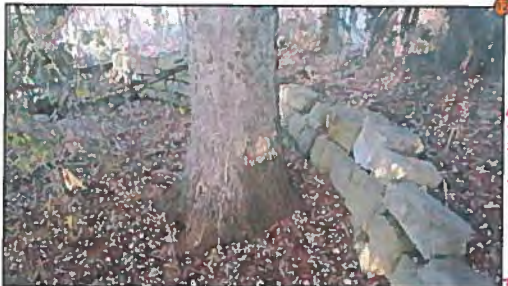
* Feature #12: Ashlar limestone wall (listed, non-designated significant feature). Part of feature impacted by proposed creek realignment.
