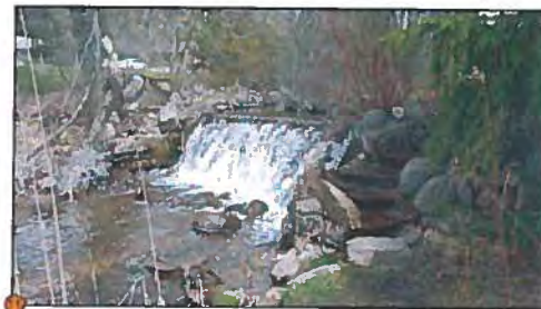
Feature #11: Fieldstone weir with steps and ashlar stone terrace wall (listed, non-designated significant feature). Feature is a substantial barrier to fish passage and limiting factor in overall channel function and health. Feature to be taken off-line/disconnected from active flow as a result of channel realignment. Feature will be maintained in landscape but will be impacted by loss of flow
