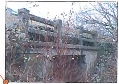
Feature #2: Reinforced concrete road bridge railing (potential significance). Feature to be modified to accommodate road widening works.
