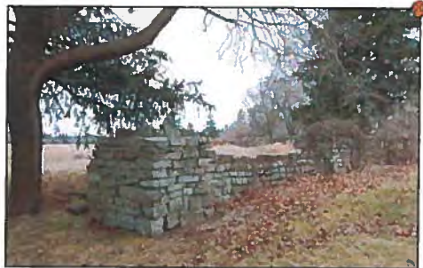
Feature #20: Ashlar dry stone wall (listed, non-designated significant feature). No impact to feature anticipated
