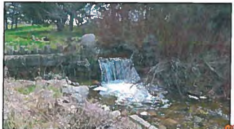
Feature #14: Fieldstone weir with cut stone terrace wall (listed, non-designated significant feature). Feature is a substantial barrier to fish passage and limiting factor in overall channel function and health. Feature to be taken off-line/disconnected from active flow as a result of channel realignment and maintained within landscape. Potential for overflow channel to reconnect during times of high-flow
