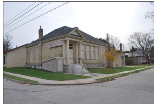
Blocking of window openings should be avoided
